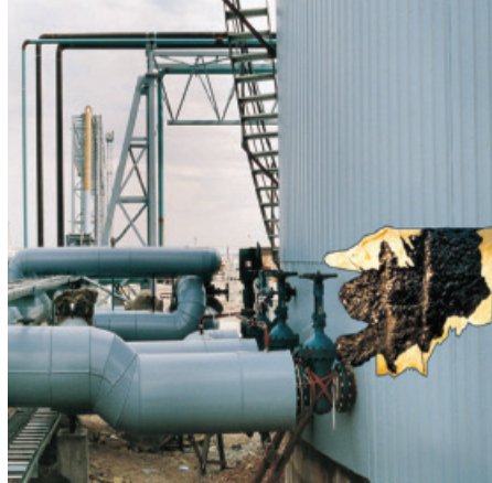
Tank insulation that has been impregnated with bitumen should be replaced.
