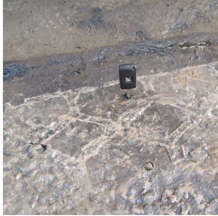
Deterioration and softening of asphalt due to fuel spillage.
