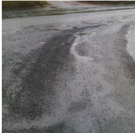
A damaged road that suggests the defects could be due to a poorly mixed asphalt.
