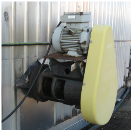
Electric driven agitator side mounted on a bitumen storage tank.
